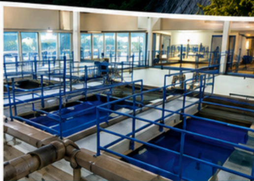
STATION DE POTABILISATION MODERNE
